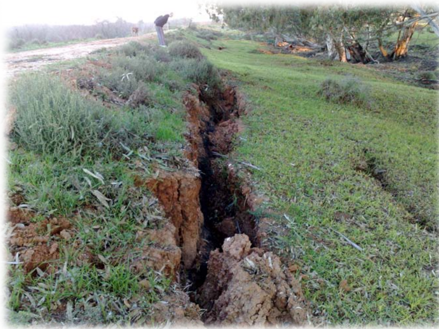
Figure 12: Levee bank cracking, Lower Murray, South Australia 2009
