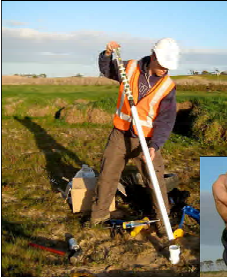
Plate 19. Installation of moisture probe into PVC access tube at Campbell Park.
