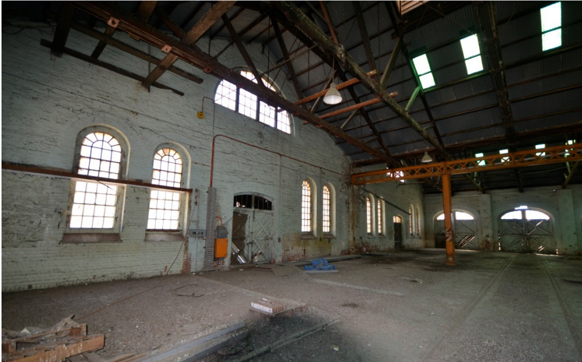
Old Bulk Store – Interior – note original central metal web truss and support columns
