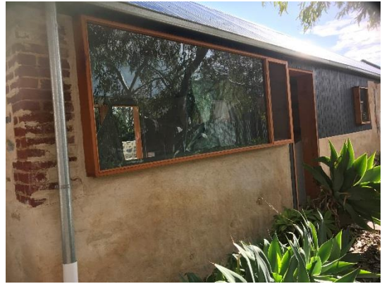
Building 2. East elevation of Building 2. Note half-height walls with windows and timber panelling above.
