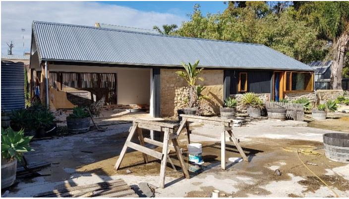
Building 2. West elevation of Building 2 (stable). Note limestone panel with open end kitchen area and half-height bluestone walls. July 2017.
