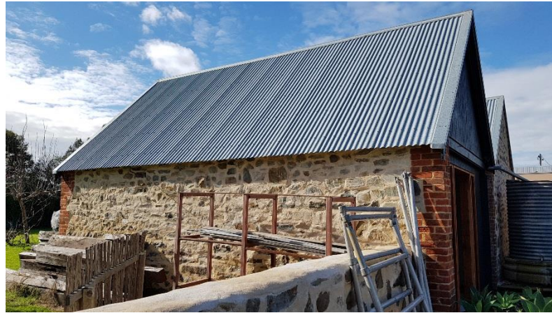
Building 1. West elevation. Note double gable ends of the south side of the building with timber infill and bluestone cladding. July 2017 Source:DEW
