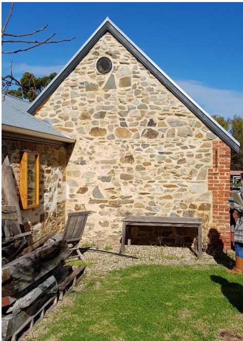
Building 1. North elevation. Note gable end with random bluestone stonework with redbrick quoins. July 2017 Source: DEW
