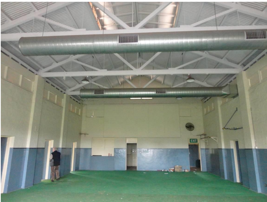
Interior of Drill Hall Building (main hall with doors to side rooms) (Grieve Gillett 2014)
