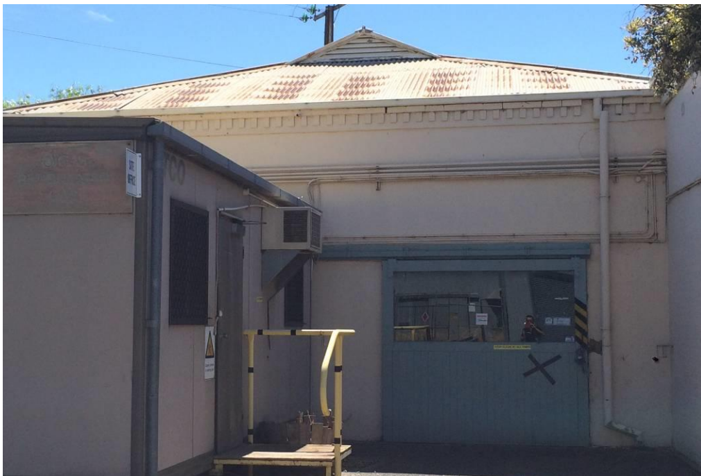
Former SAGASCO Gasworks, Brompton – Building B102 (Former Reticulated Gas Workshop), view from SE end (2015)
