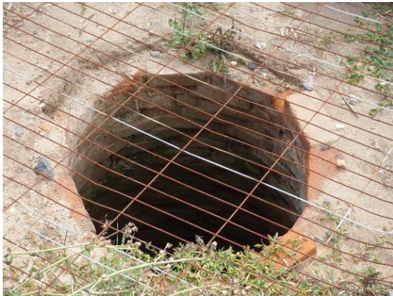
Uncovered well 23 November 2017 Source DEW
