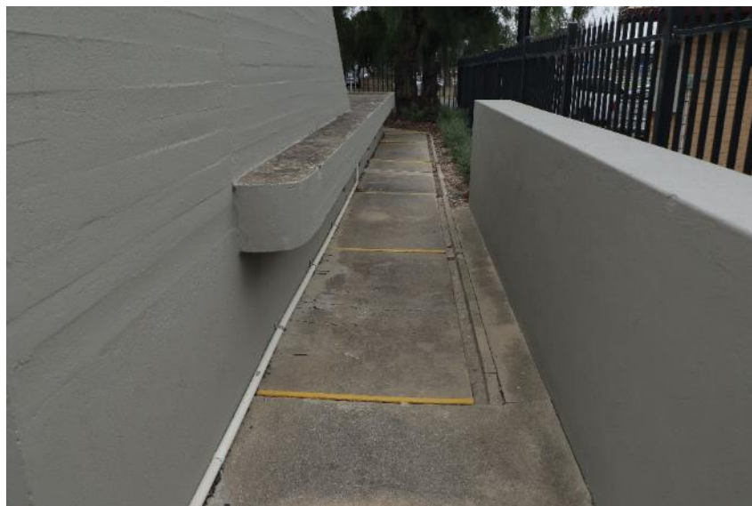
Side view showing original cement paving and integrated drain DEW Files 4 February 2021
