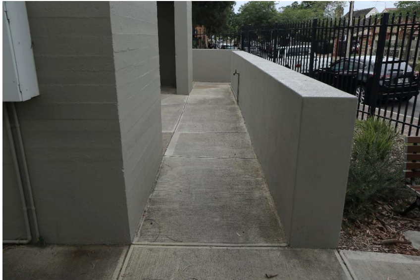
Front entrance showing baffle wall and new concrete paving DEW Files 4 February 2021
