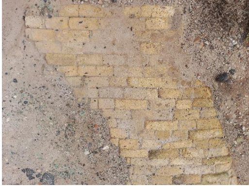
Paved firebrick working floor
