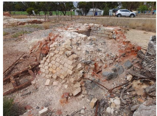
Chimney of Smelter A showing collapsed firebricks Source: DEW Files 1 March 2022
