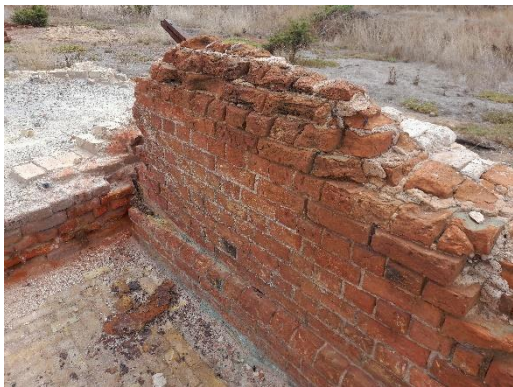
Chimney of Smelter B showing eroded, previously exposed upper courses
