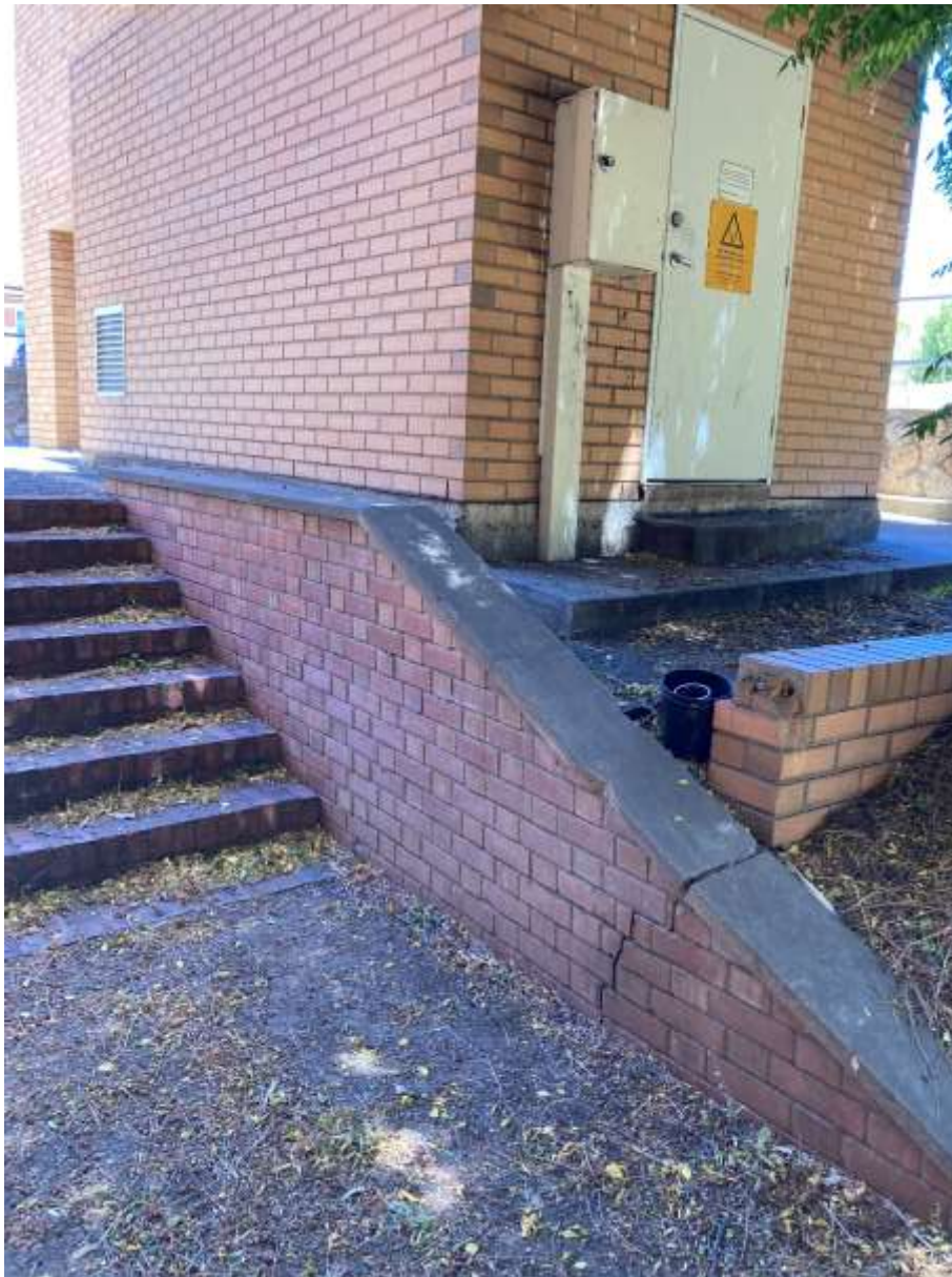
Steps to sunken garden (left), foot of tower (top left) and plant room (top right)
