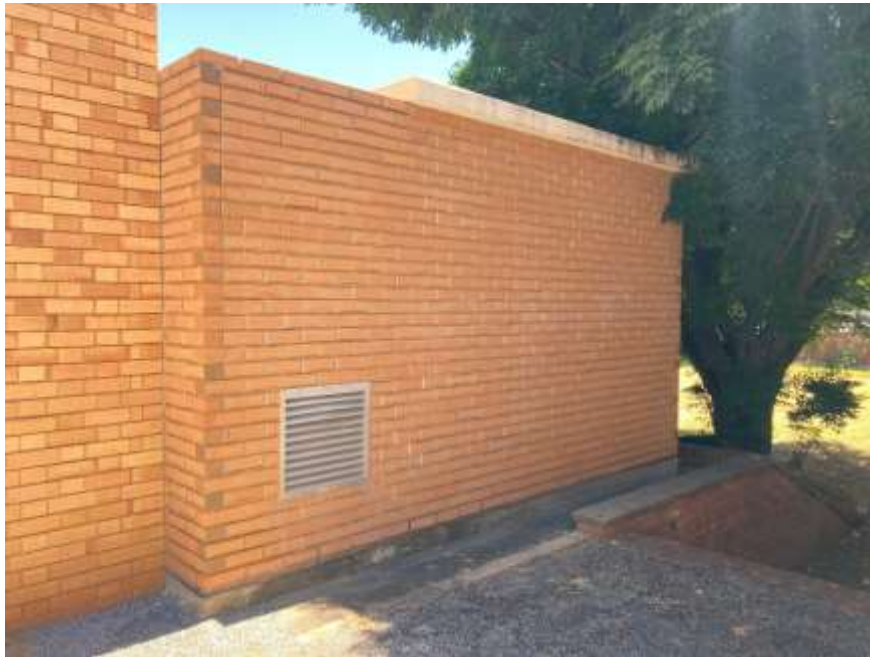
Side view of 1980s plant room and steps to sunken garden (lower right)
