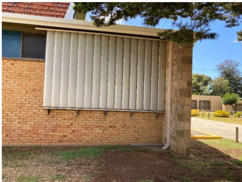
Adjustable aluminium louvres on western elevation, shading baptistery window Source: DEW Files 28 January 2021
