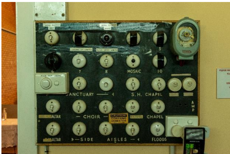
The 'Palladium-like' switchboard
