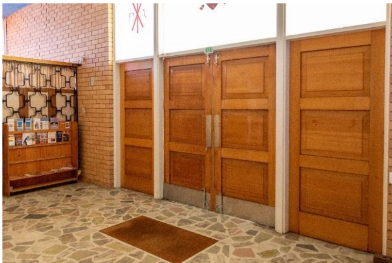
Narthex showing main entry doors, with Italian and Angaston marble floor in a matrix of terrazzo
