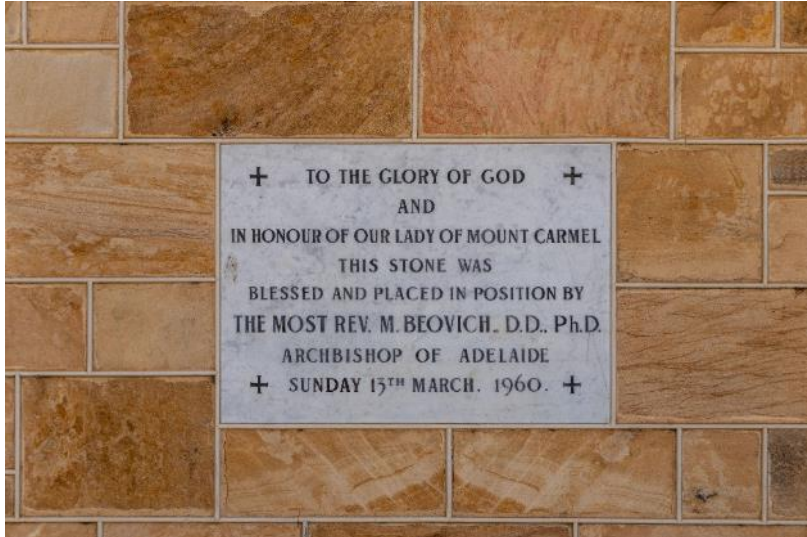
Foundation stone showing sawn basket range stone facade Source: DEW Files 28 January 2021
