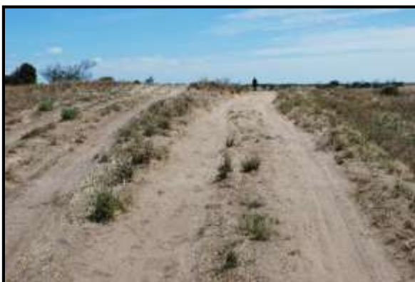
Figure 15: Degraded track (right) with new track (left)
