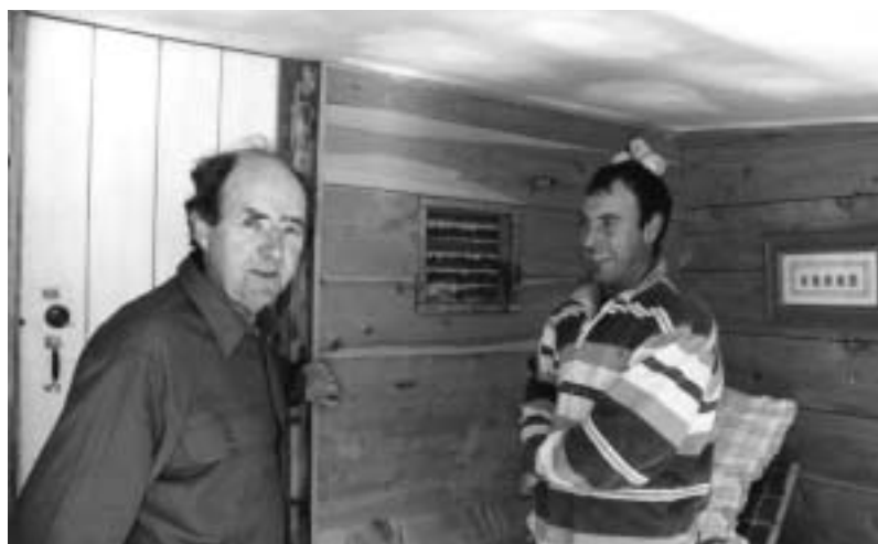
John Fenton and Steven Clements in front of the square of internal wall left unlined to reveal the original laths.
