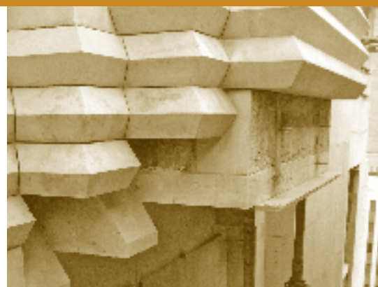
Several stones were removed from under the northern projecting abutments prior to new replacement stone being installed.
