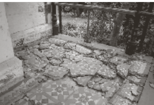
Korra Weera, Marden, veranda tiles before repair
