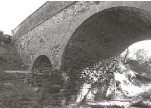
Ross Creek Bridge, Kapunda, before repair
