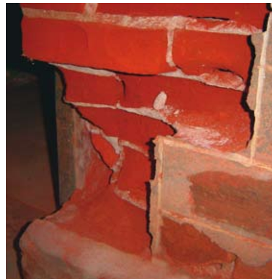
Different materials deteriorate at different rates - these bricks are an easy target for salt damp.
