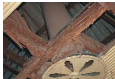
Termite damaged roofing timbers, Morgan Railway Station (2007).
