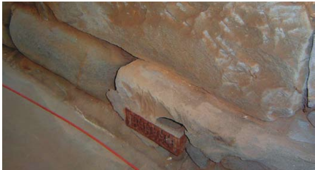
Concrete slab next to stone wall – moisture is forced up the wall instead of evaporating from the ground
