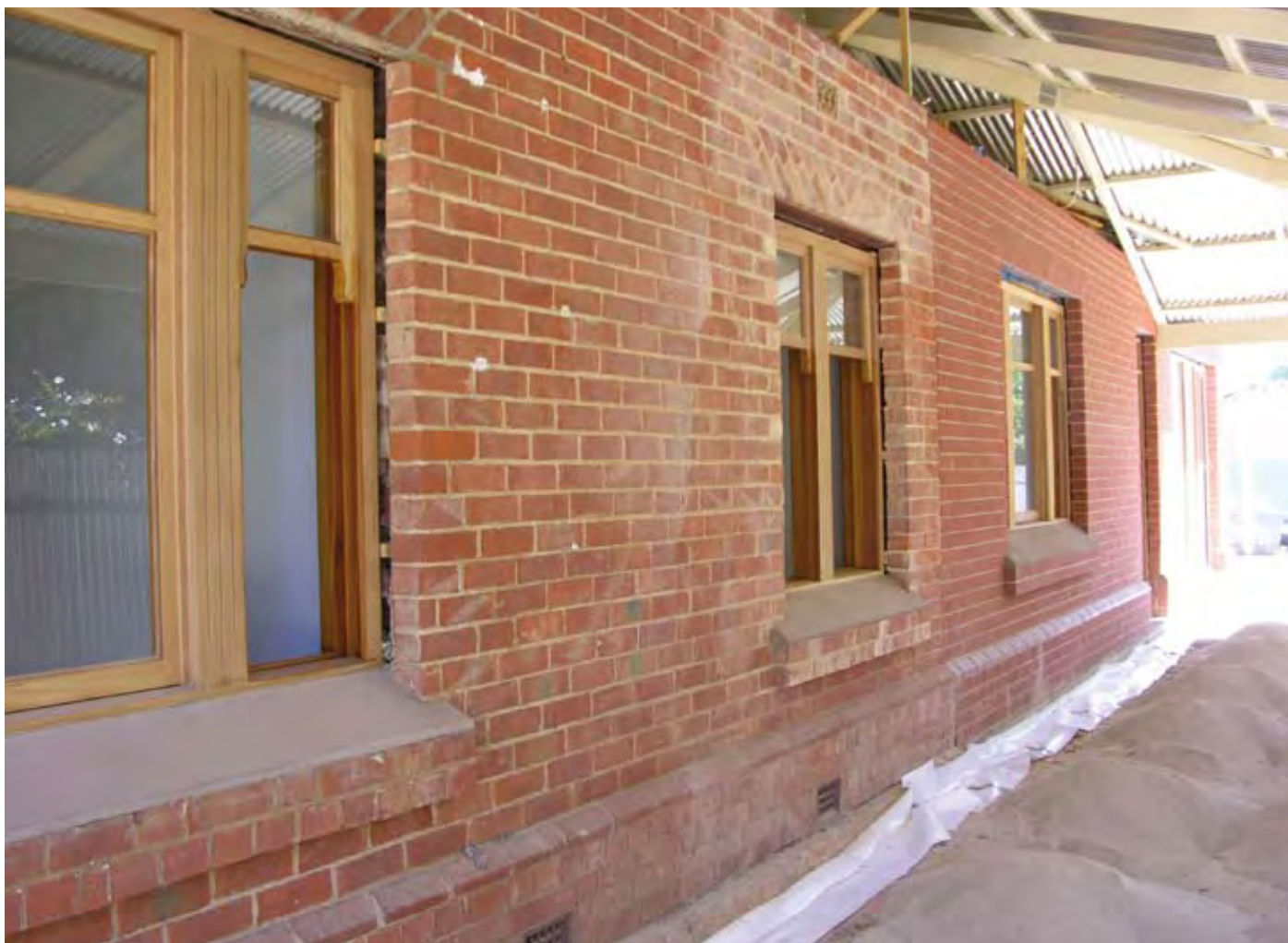
Northern wall of house after renovation showing new window opening created in original section, as well as new rear addition. While in this example the new work has been designed to blend with the original, the practice of making new work in a contrasting style is also encouraged.
