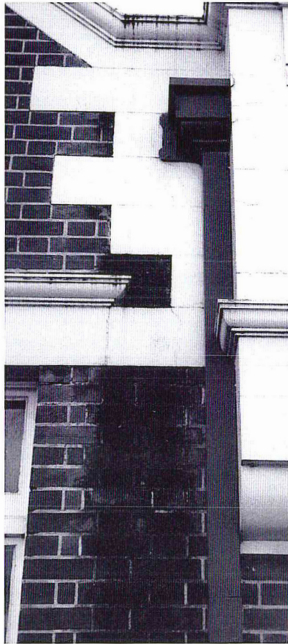
Blocked downpipe and rainwater bead causing decay of brickwork below.
