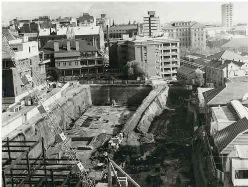
Excavation of the centre of the site during 1963 looking west to the rear of Margaret Graham and Eleanor Harrald buildings. (Source: SLSA B15535)
