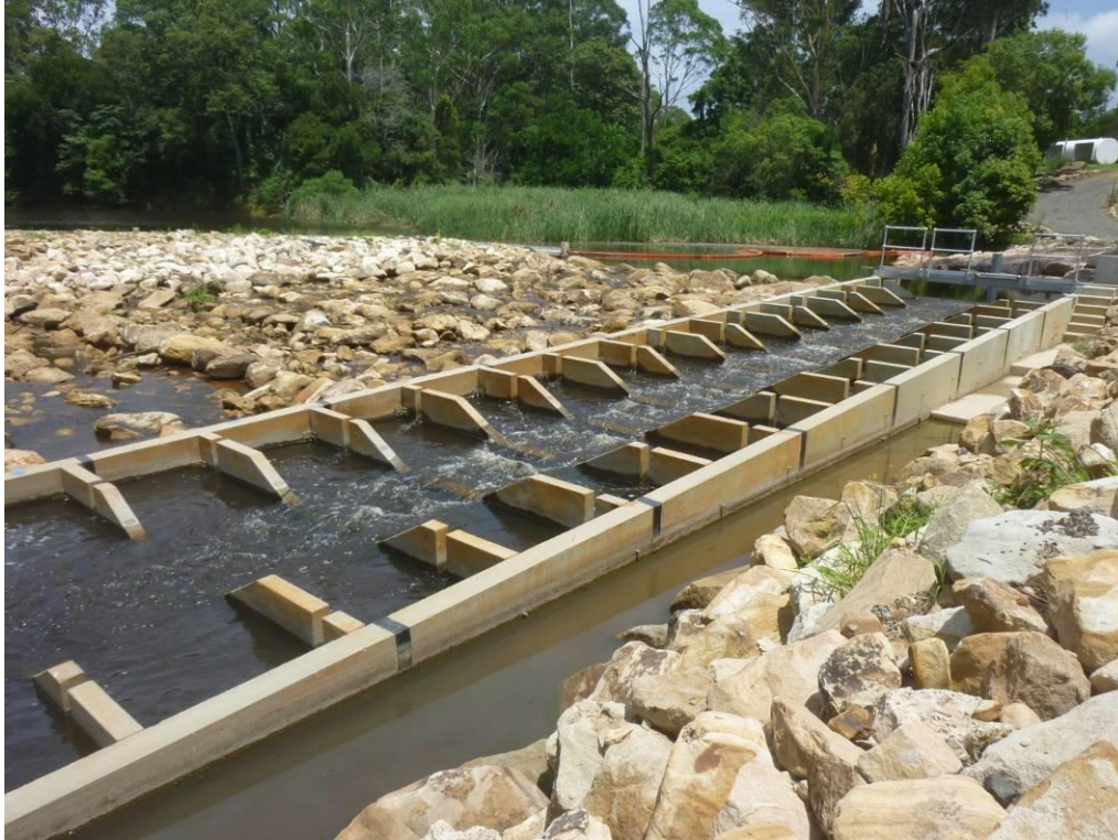
Figure 16. Example of a trapezoidal weir fishway on a coastal stream of NSW.
