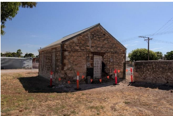
Rear entry of Ticket Office with visible degradation and old repairs.
