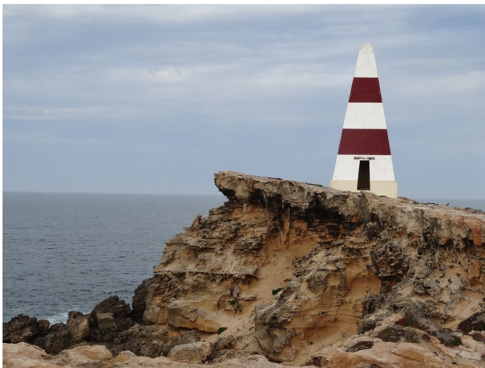
Cape Dombey Obelisk showing the tapered doorway to the internal storage area and erosion to the cliff face, 2016.
