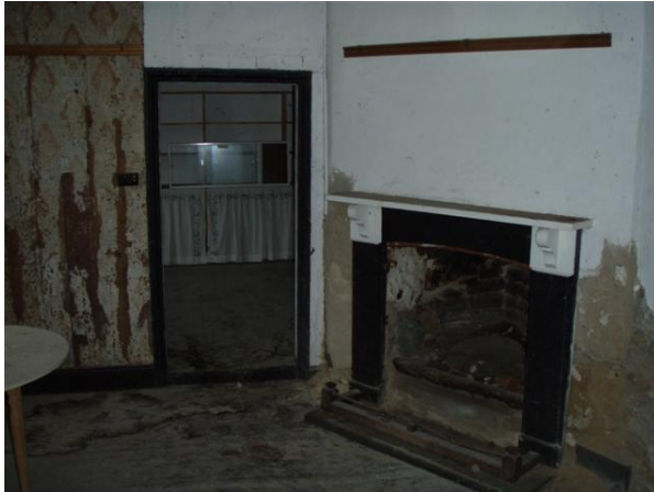
Interior of Bush Inn prior to conservation work showing one of the fireplaces, c.2008.
