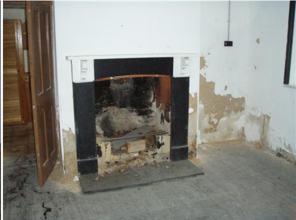
Interior of Bush Inn prior to conservation work showing one of the fireplaces, c.2008.
