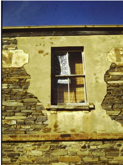
Northern window of the upper storey of London House prior to conservation in 1993.
