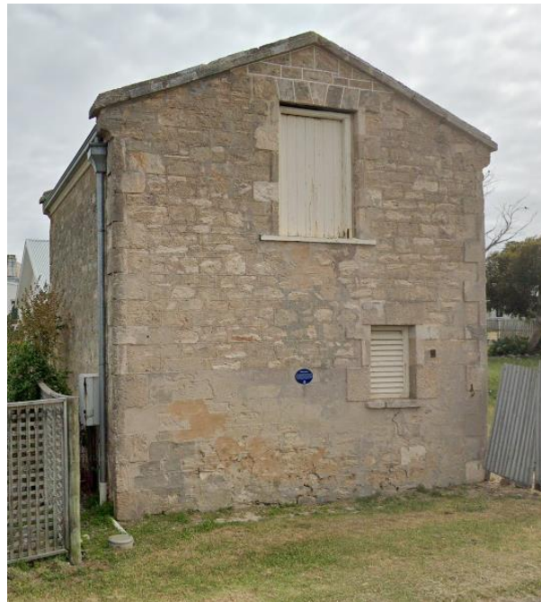
The southern elevation of the Police Stables in 2020, note the repointing of the walls.
