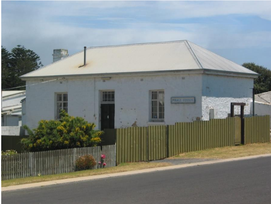
View to front of the Courthouse in December 2003. The roof sheeting has been replaced and the 'Police Station' sign is still on the building.
