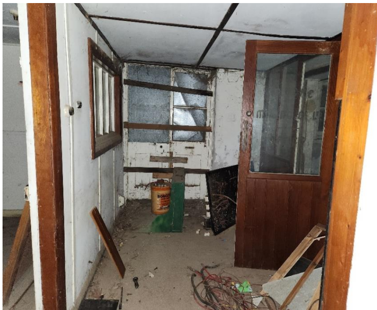
Interior of the lean-to office from the flour mill. The door in the centre leads out to Commercial Road.
