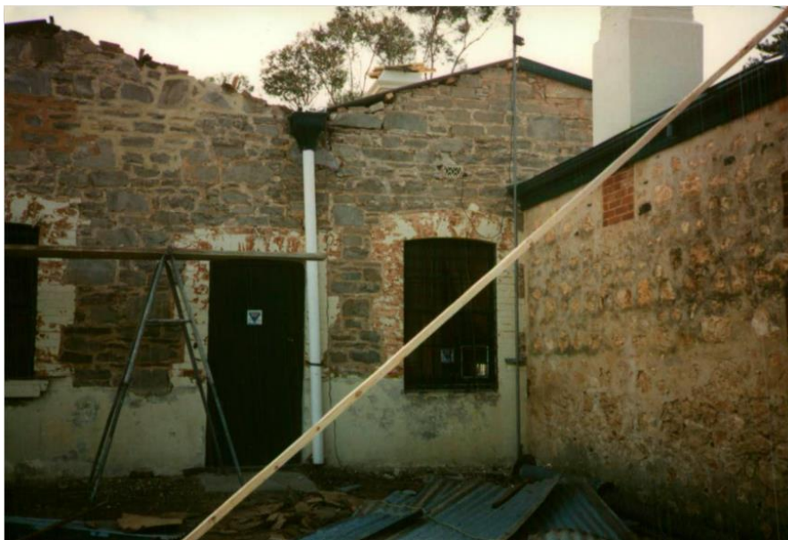
Rear of 4-6 Albyn Terrace during conservation works in the late 1990s. This photo was taken during the installation of the verandah.
