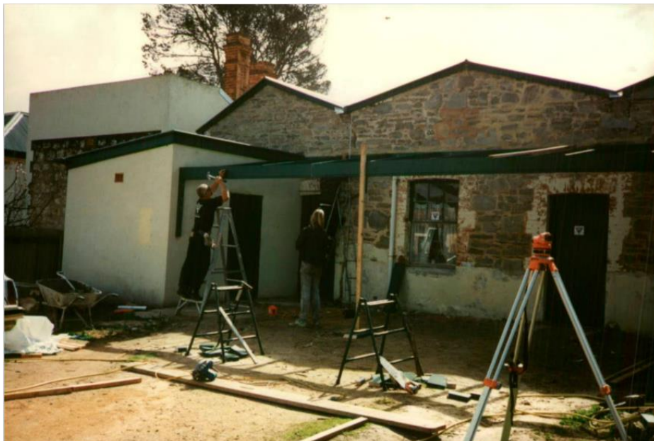
Rear of 4-6 Albyn Terrace during conservation works in the late 1990s during the installation of the rear verandah.
