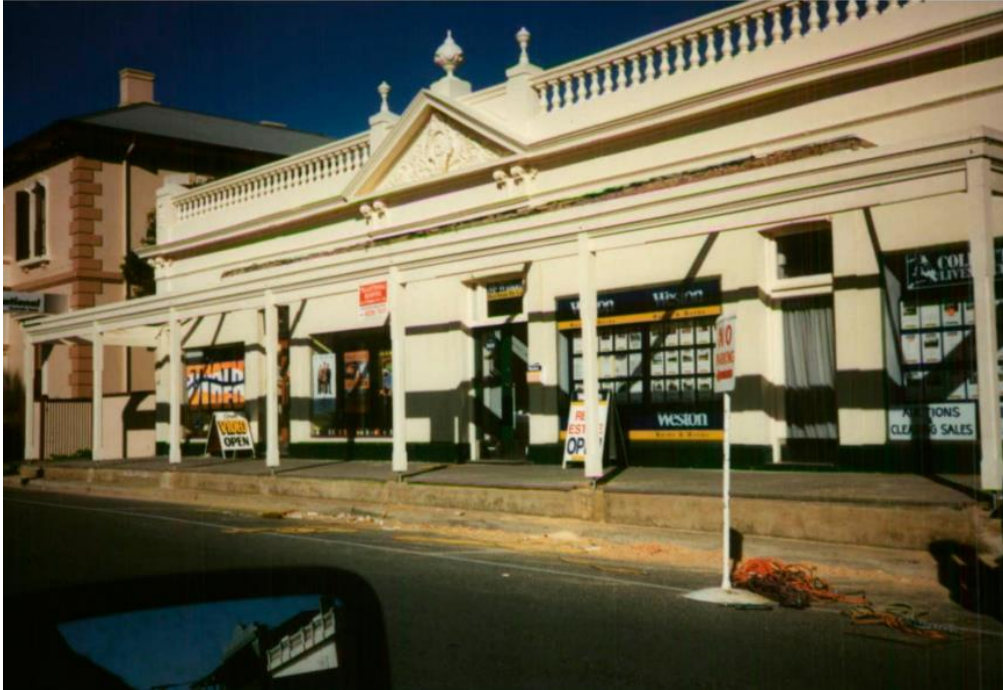
Shopfronts of 4-6 Albyn Terrace in the late 1990s during the installation of its new roof and front verandah.
