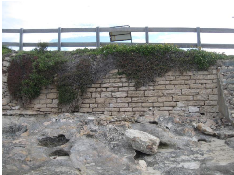
Closer view of a portion of the Seawall in front of the Royal Circus, c. 2011. Given the various repairs made over the years, the Seawall likely consists of original and non-original stones.
