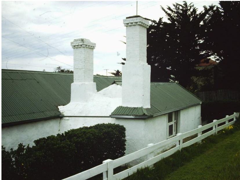
Two chimneys built of brick and stone on the c.1853 section, c.1982.
