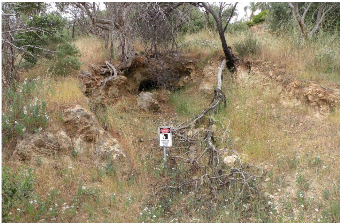
Entrance to the collapsed stone mine on Council Reserve, Lot 19
