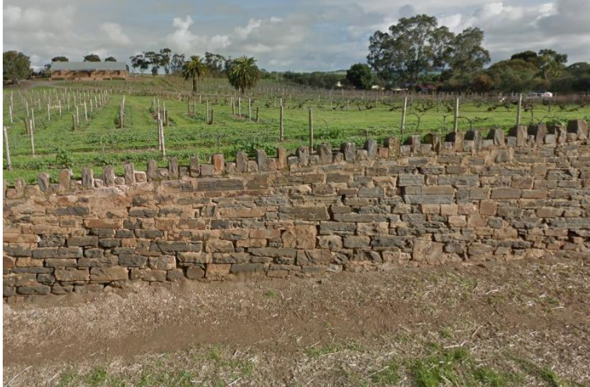
Bluestone Wall along the north east boundary of the site. Note the rubble masonry and crenelated decoration across the top.
