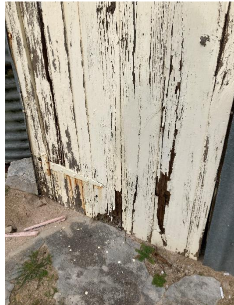
Detail of the rear door showing weather damage, 2022.
