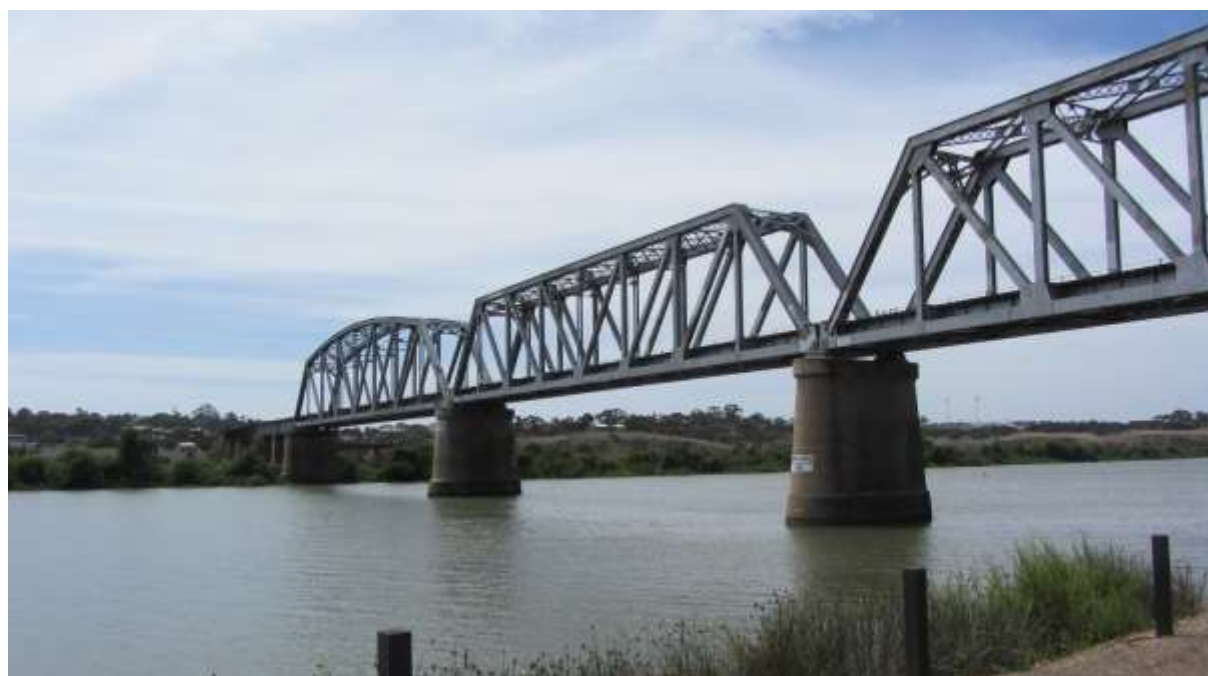
Murray Bridge Railway Bridge [Metal Truss] (SHP: 13826) Murray Bridge Transport Precinct, Murray Bridge
