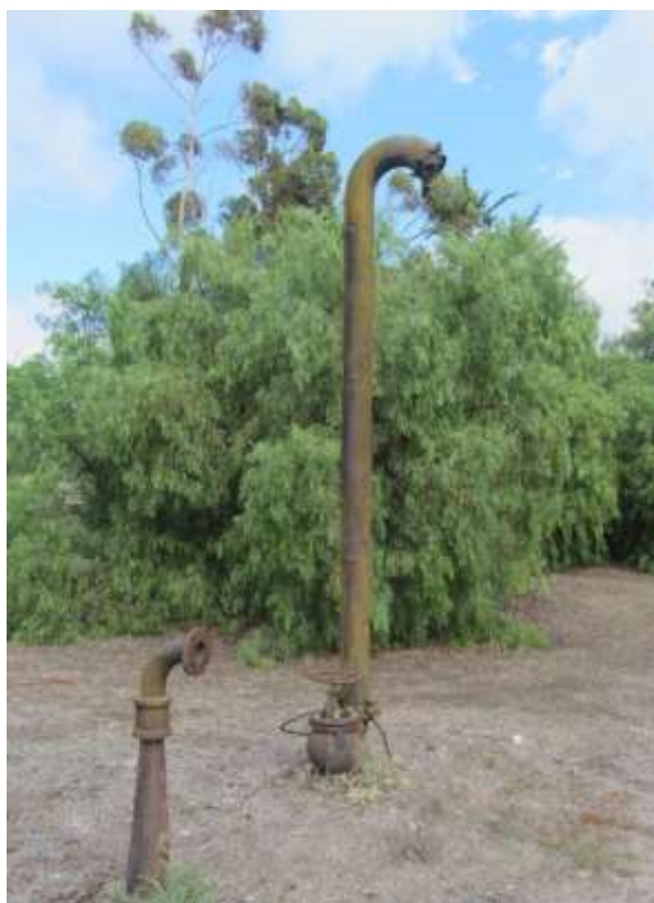
Water Column (standpipe)
