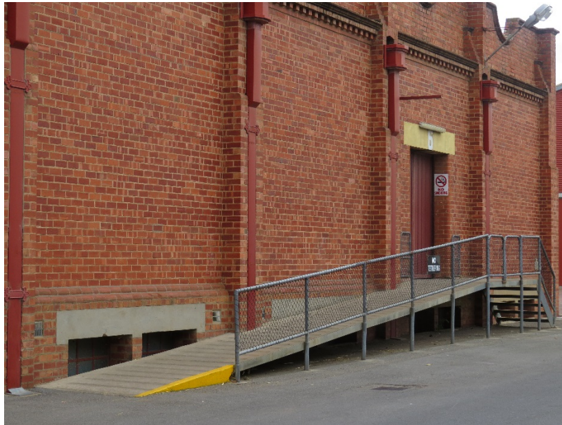
Stud Sheep Pavilion, northern addition, eastern façade showing detailing, ramp and cellar
