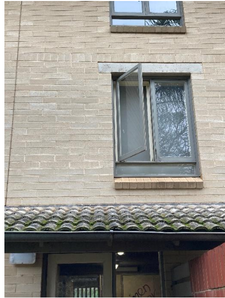
Flats showing window details, note concrete lintel, band of brick above, brick sill and concrete tiles to roof.
