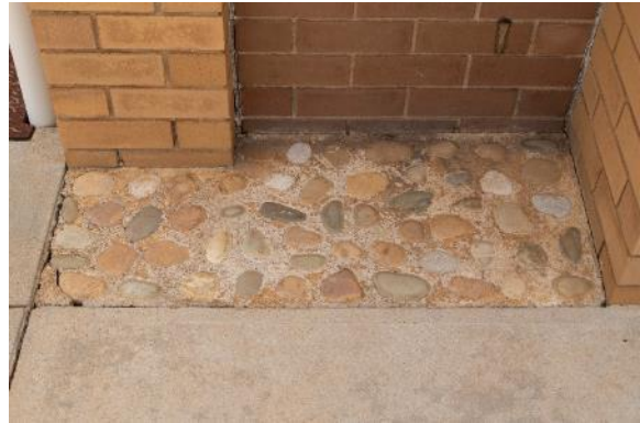
Pebbles in concrete between front elevation and footpath
