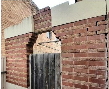
Side gate showing subsidence and missing pointing
