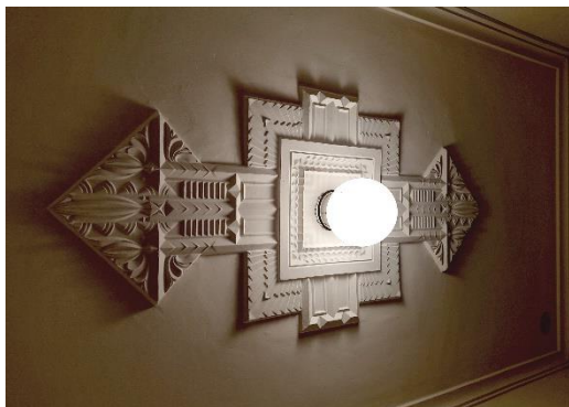
Typical ceiling rose
