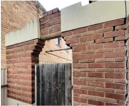
Side gate showing subsidence and missing pointing
