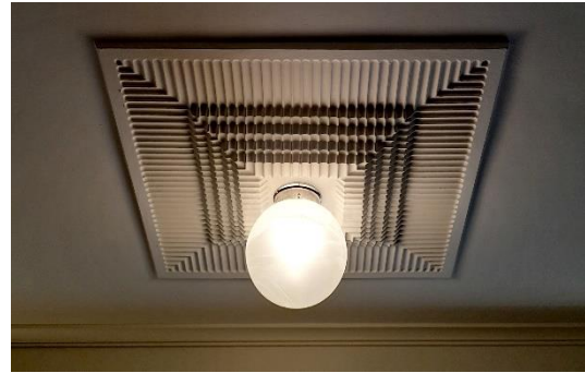
Typical ceiling rose
