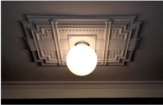
Typical ceiling rose
