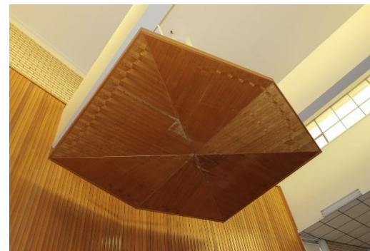
Underside of baldachin showing water damage
