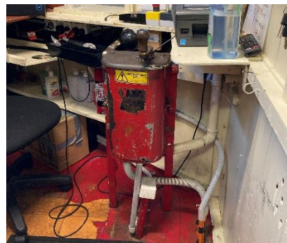
Carousel controller (ex MTT tram controller).
