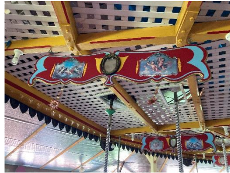
Sweeps, quarterings, lattice ceiling [original fabric] with drop panels [not original fabric].
