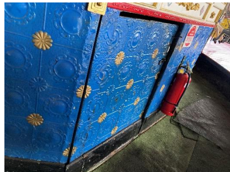
Pressed metal cladding of lower centre console and access door.
