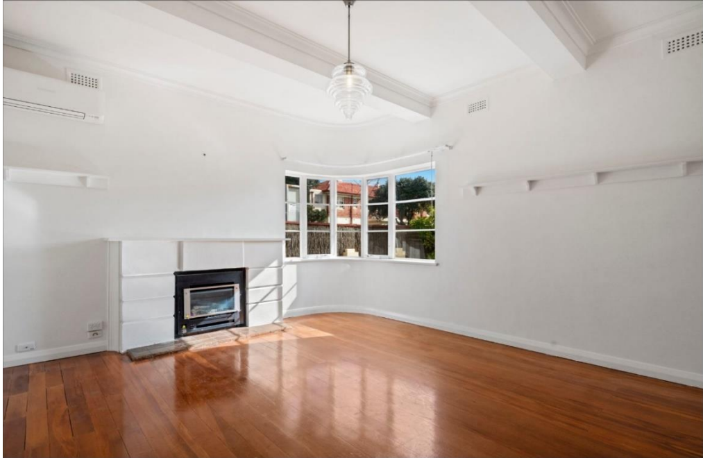
Lounge room of western downstairs flat, showing original fireplace, shelving and concrete beams supporting second storey floor.
