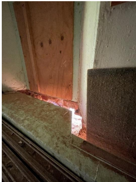
Internal view of the hole on the western wall.
