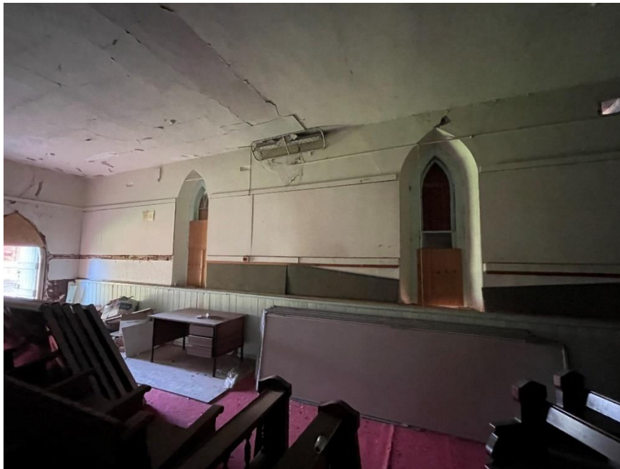
The interior side of the western wall showing two of three extant windows. The crack in the ceiling demarcates the original part of the building and the extended part.
