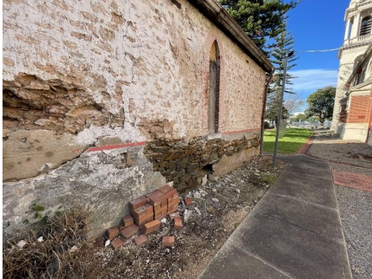
Part of the western wall of St Patrick's Schoolhouse showing part of the bluestone base courses.
