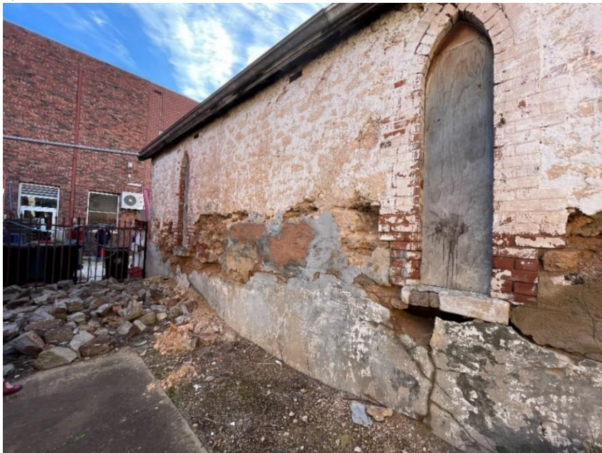
Part of the western wall showing considerable damage to the limestone walls, including a hole under the middle window.
