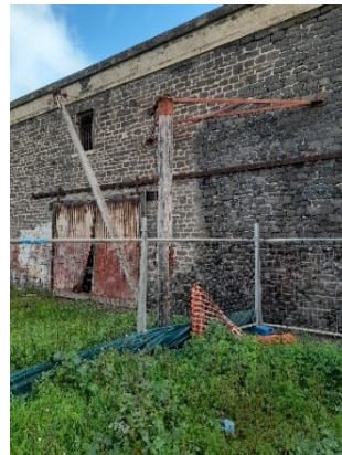
Derrick crane in vicinity of former Central Slip, attached to Fletchers Slip Precinct (SHP 11872)
