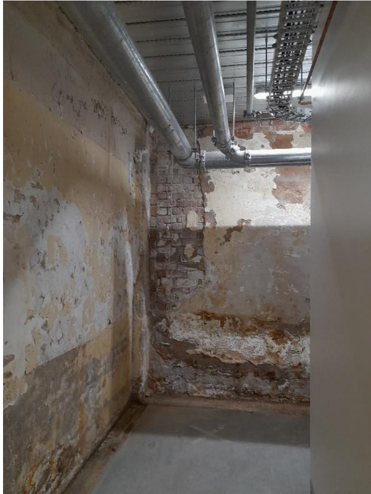
Rising damp damage in the basement.
