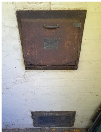
Incinerator furnace and ashpan doors
