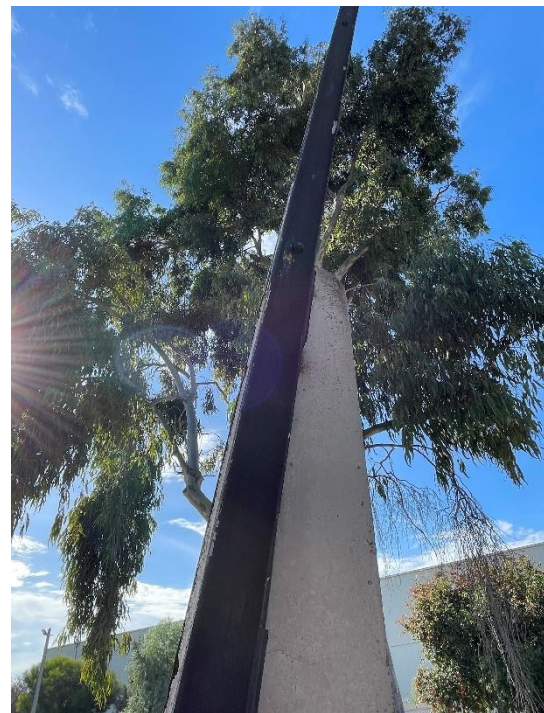
Righthand side of the 1924 Stobie pole showing one of the steel beams.
