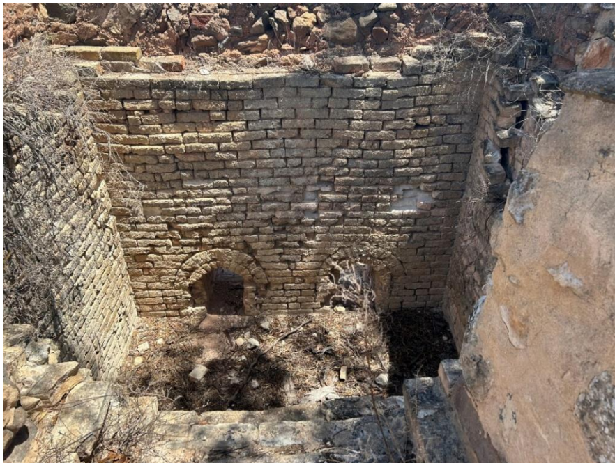
Interior of the western lime kiln. This kiln retains its double-layered fire brick lining.
